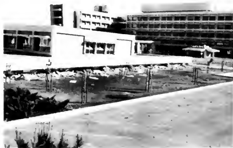
Photo 35. Psychiatric Unit, of which the first story collapsed. Los Angeles County Fire Department photo.
